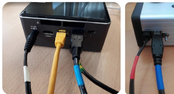
Figure 5.8 – Color marked wire connection to the computer unit (left) and to the device (right).
