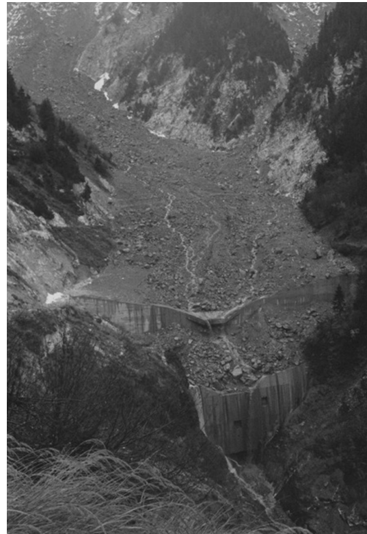
Figure 1.7 – Bon Attrait deepseated landslide and its double consolidation dam ( \approx 100m wide, from left to right bank wings), Ravoire de Pontamafrey torrent (73) Fr., construction: 1968-1970 (photo Nov. 1979 by JL. Boisset courtesy of ONF-service RTM 73)
