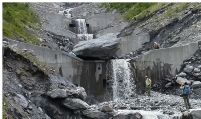
Figure 1.10 – Huge boulder stopped on the check dam series of the St. Antoine torrent upper basin (73 – FRA.) – 2014 (photo courtesy of S. Carladou)
