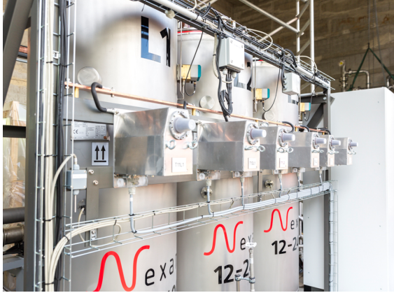
Figure 1.22: Picture of the R-SFCL from the Ampacity project installed in Essen, courtesy of Nexans®.
