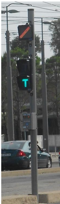
Signal de Manoeuvre
