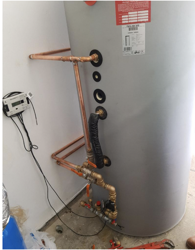
FIGURE 5.16: Photography of the newly installed boiler
