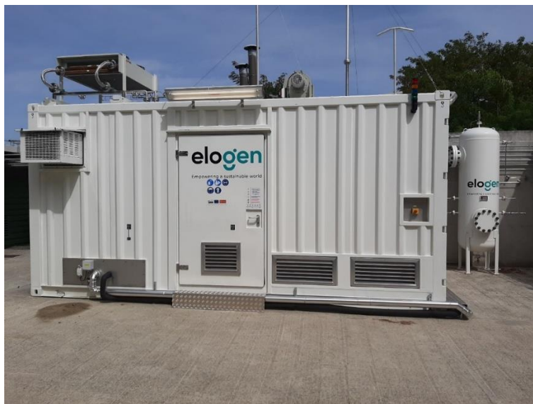
Figure I-12. A PEM electrolyser unit container. Courtesy - Elogen.
