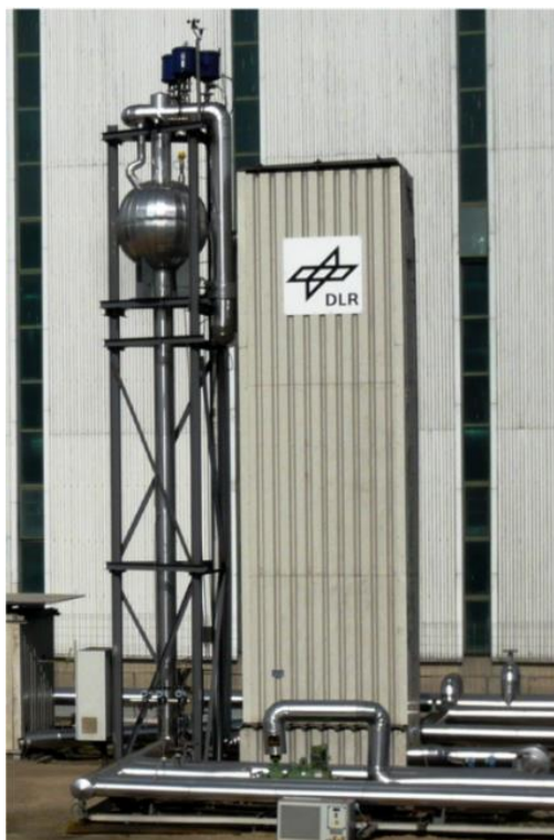
Figure 13. Insulated PCM test module at the test site in Carboneras, Spain [17]
