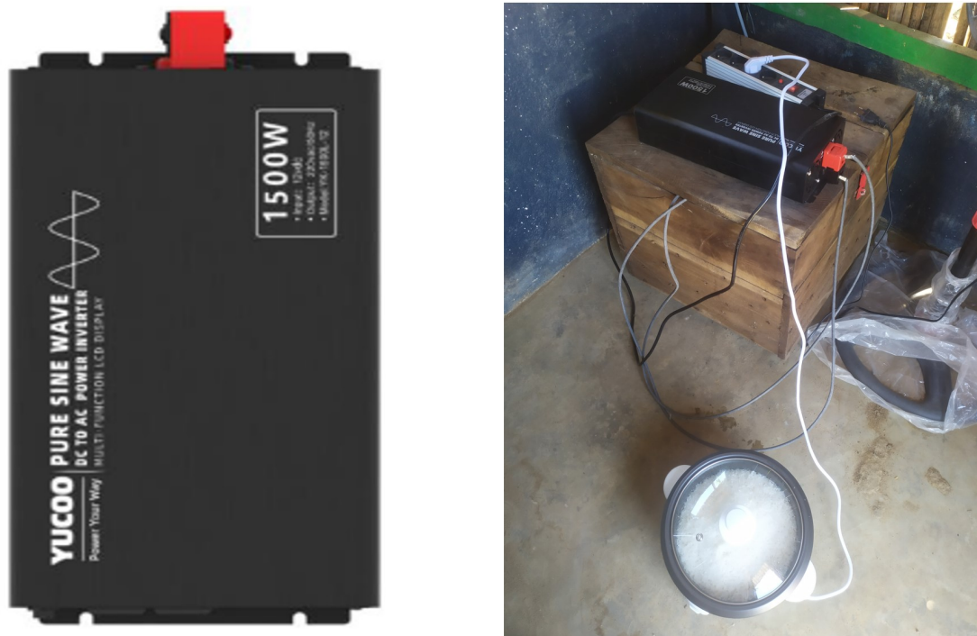
Figure IV.16: Rice cooking using an AC inverter on the microgrid.
