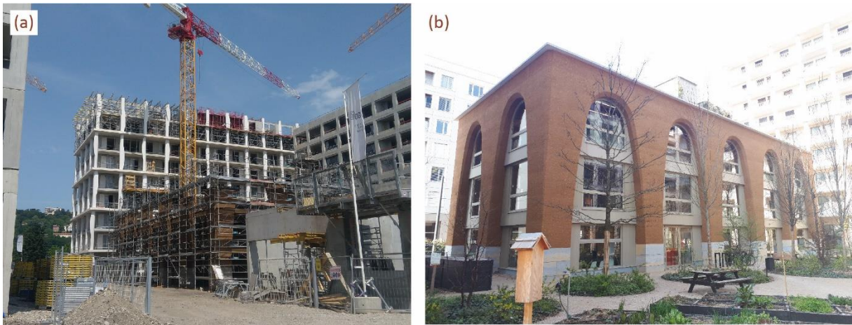
Figure 0.1: (a) Picture of the project taken during construction and my internships; (b) Picture of the finished building (source: author)
