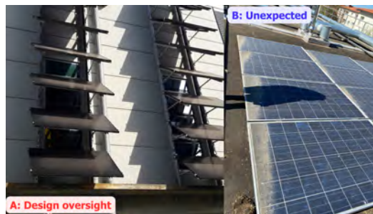
Figure 3: Some example of unexpected shadows. A is mostly a design oversight, while B is unexpected build-ups.
